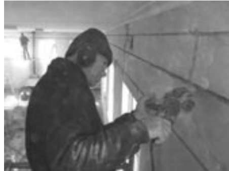
Brother Joseph cleaning the cuts in the walls which will be reinforced with metal spiral cable to repair the severely cracked walls in the Seminary Refectory.
