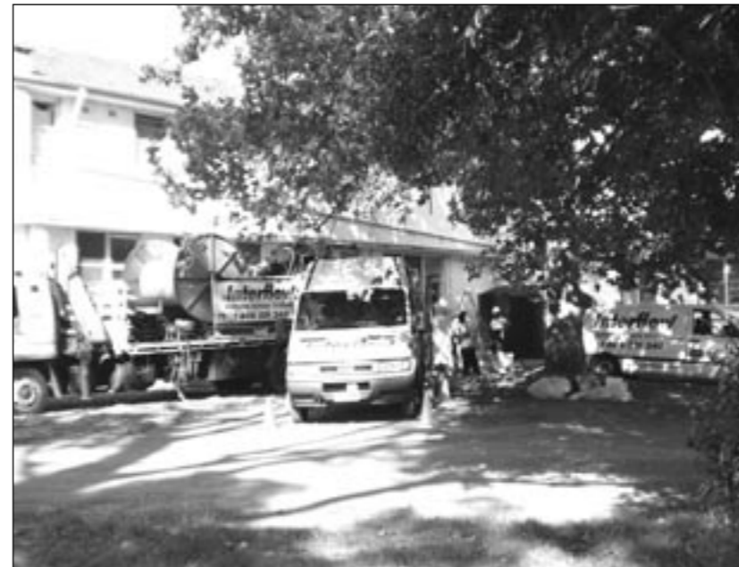
The old clay sewer pipe is "lined" with an internal PVC pipe, eradicating drainage problems and allowing work to begin on the structural repairs of the buildings foundations.
