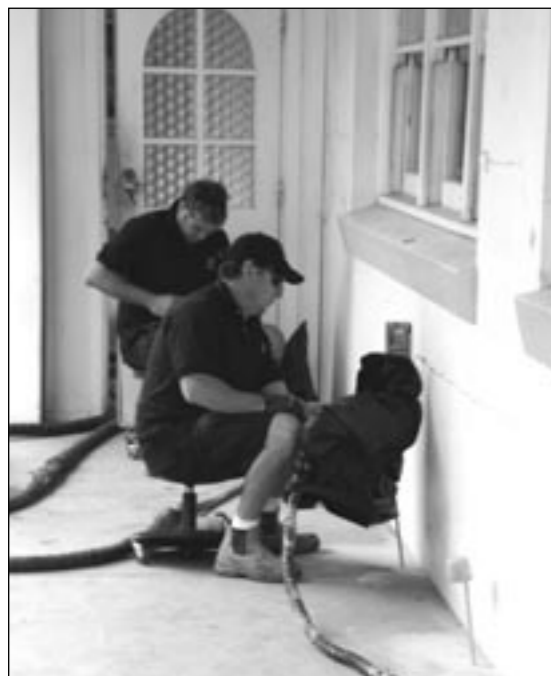
After drilling beneath the building foundations, these workmen seem to "sit idly – however they are literally raising the two storied Mater Dei Wing by pumping thousands of dollars of "high-tech mud" into the ground.
