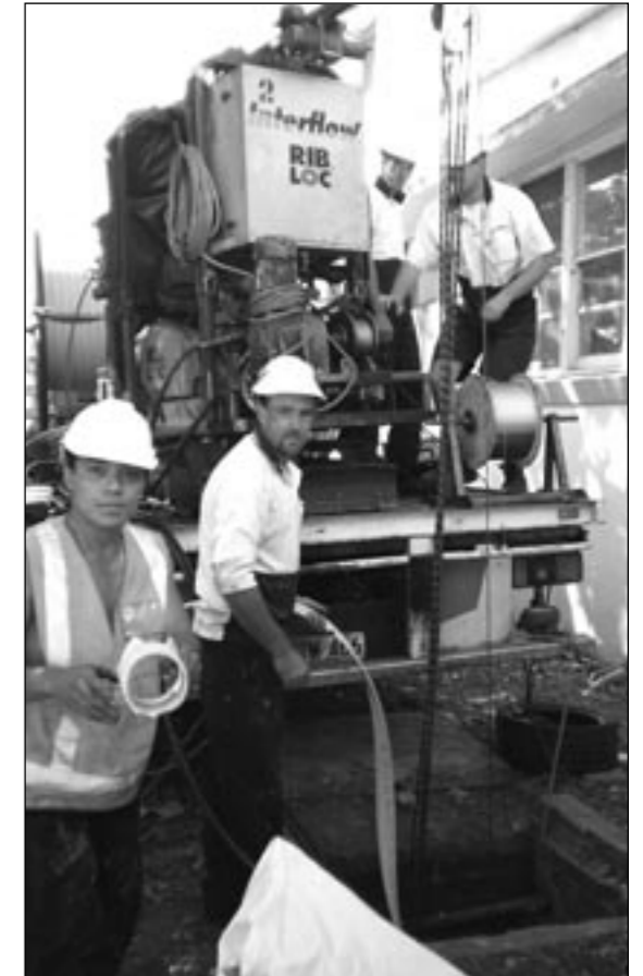
Some workmen pose with the tools and product of their trade as they repair the buildings old sewer lines
