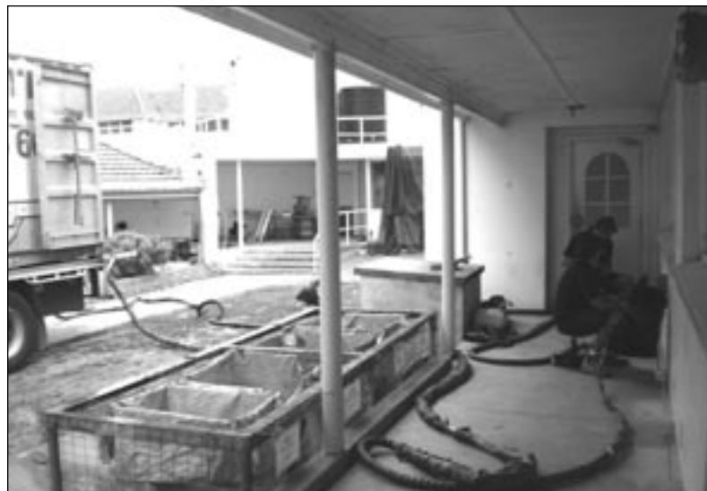
The foundations of Mater Dei Wing, at the Kitchen, are being supported and raised by the injection of high-tech "mud" (a polyurethane mixture) in a process called "mud-jacking."
